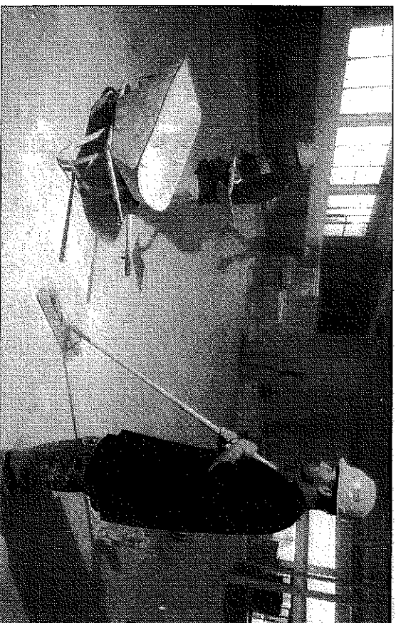
CLEANUP CREW: Teen workers Justin Wallace, left, and Scott Escoc, both 17, employed through the Mentoring and Partnership for Youth Development program, sweep a grocery store in the Lincoln Crossing construction site on Lincoln Avenue in Pasadena on Friday.
